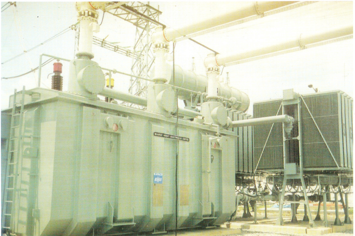
180 MVA 275/132/11kV 3-Phase Auto transformer at Skudai S/stn , Malaysia
