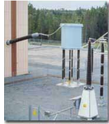
Air-core smoothing reactor in the FennoSkan HVDC transmission
